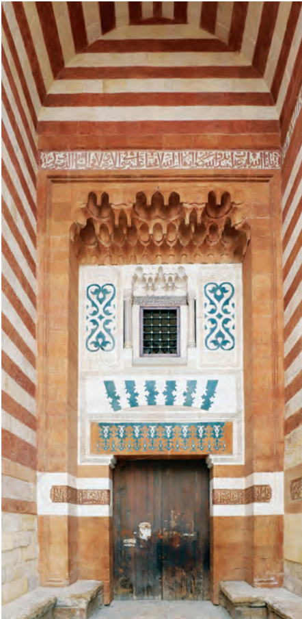
Above: View of the upper part of the mosque's east elevation with chiselled gypsum plaster openings and upper inscription band (AKTC Conservation Team, 2020).
