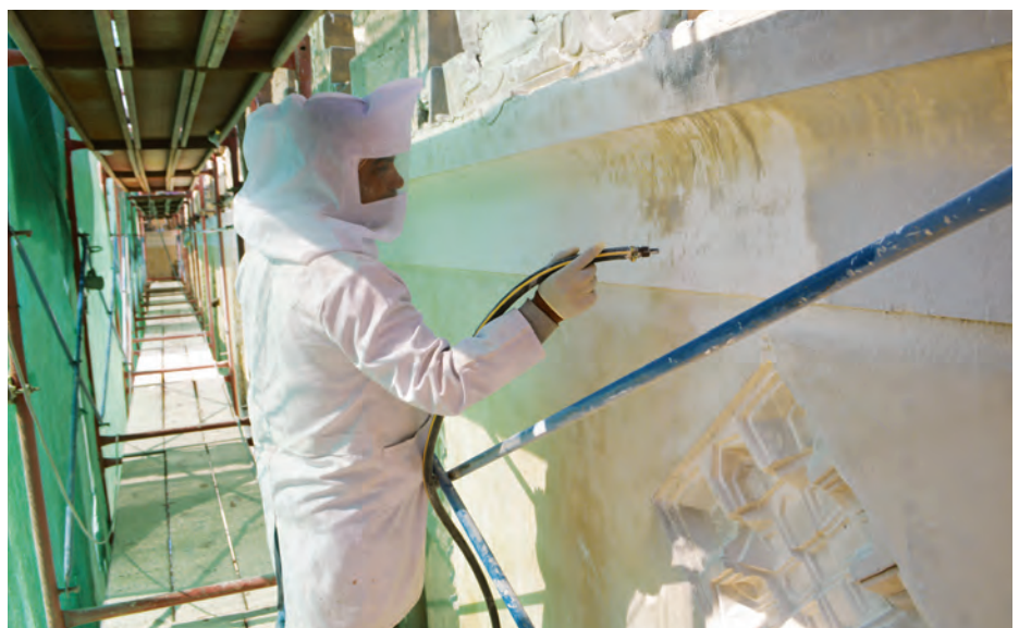
Above: Applying clay poultices soaked in ammonium carbonate below the cornice of the prayer hall (AKTC Conservation Team, 2019).
