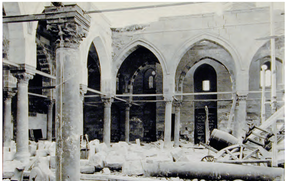
Right: The Maridani Mosque's courtyard arches under reconstruction by the "Comité" (Bulletins of the Comité de Conservàtion de l'Art Arabe, 1896).
