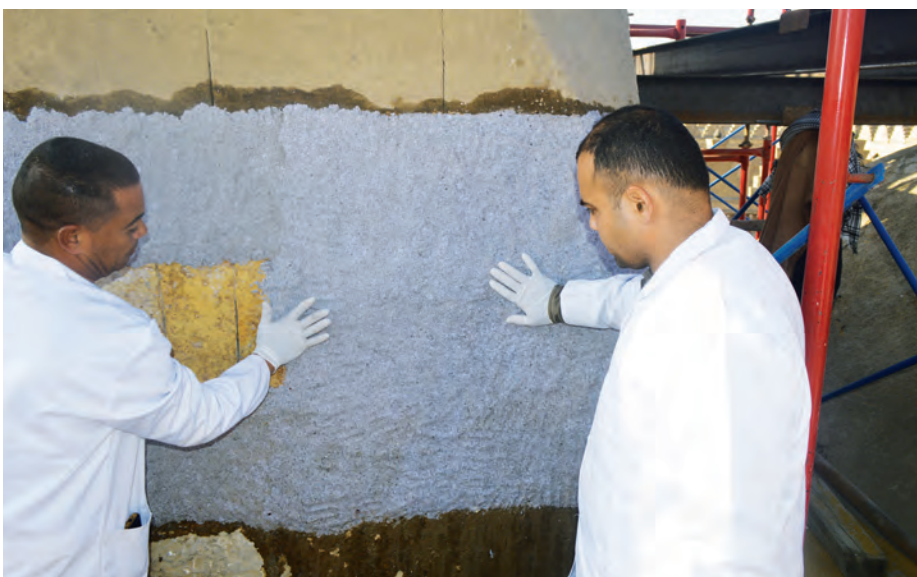
Above: Manual brush cleaning of the arch's voussoirs on the upper section of the external walls (AKTC Conservation Team, 2020).
