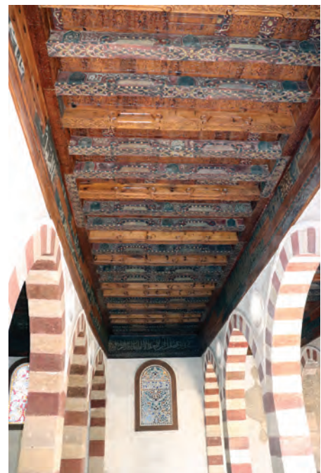
Above: View of the decorated ceiling of the prayer hall showing the combination of painted and plain coffers, the latter having been left intentionally undecorated by the Comité (AKTC Conservation Team, 2020).
