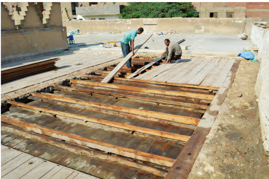
Left: Exposed structural timber and boards on the roof of the Maridani mosque during repairs (AKTC Conservation Team, 2020).
