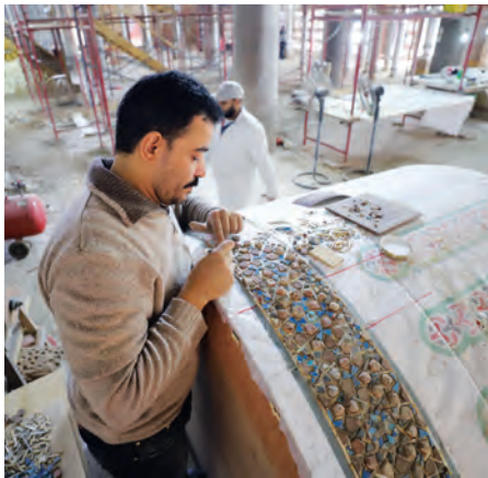
Above: Partial rectified elevation of the mihrab niche with the mapping of the marble mosaic to identify the extent of repairs and reintegration (AKTC Conservation Team, 2020).
