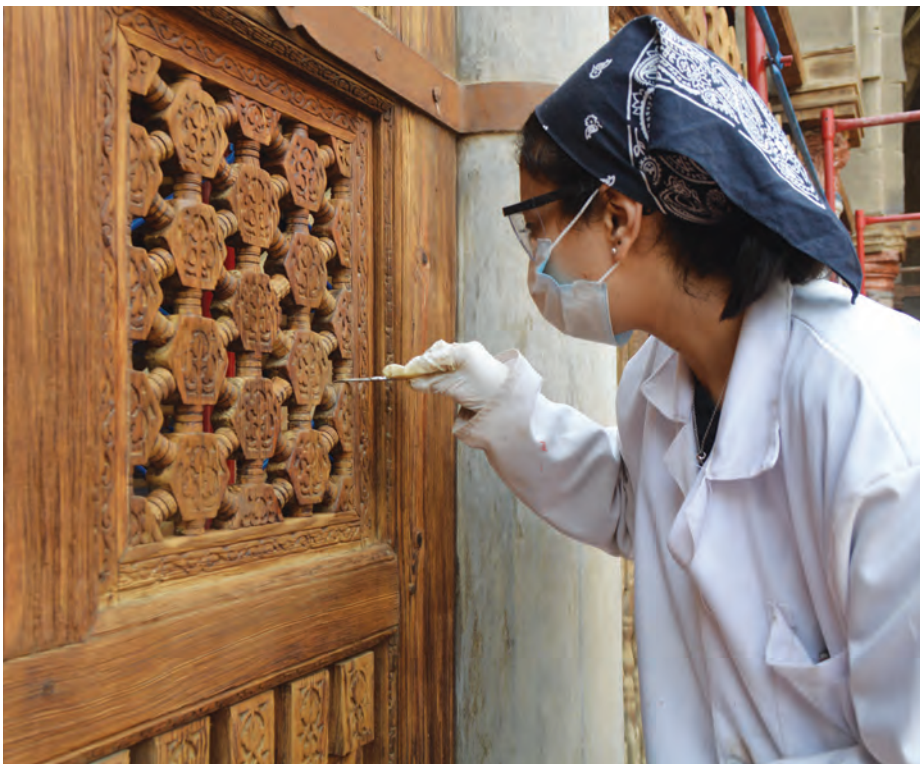
Above: Replacing lost wooden elements and decorative inlays to reconstitute the complex geometric design of the prayer hall's minbar (AKTC Conservation Team, 2020).
