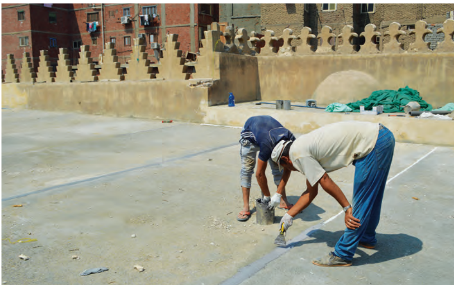
Above: Application of the first mortar screed in between expansion joints (AKTC Conservation Team, 2020).
