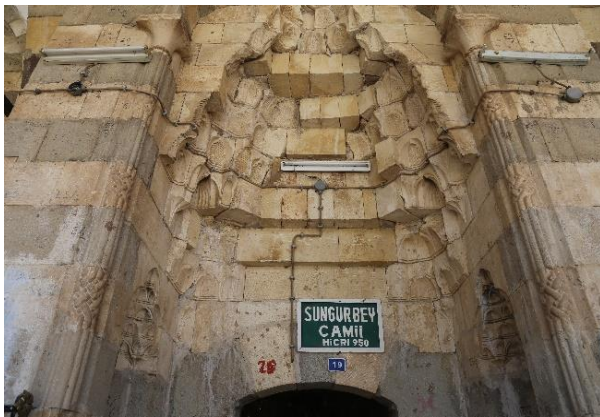
Figure 3. Assembly problems of the crown door
