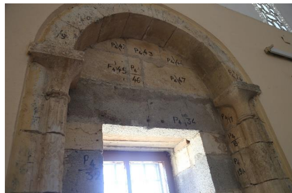
Figure 6. Cracks in the lintel above the window.
