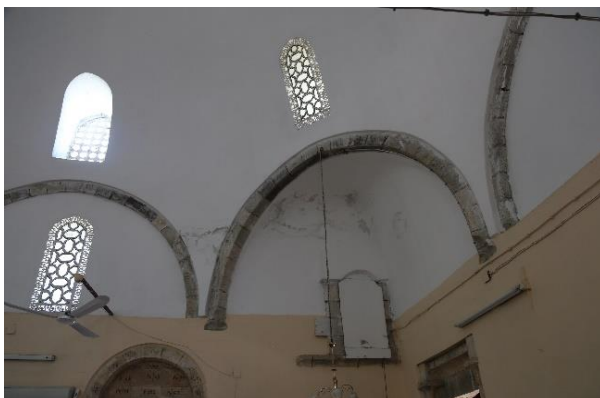
Figure 5. An example for Insulation problem.
