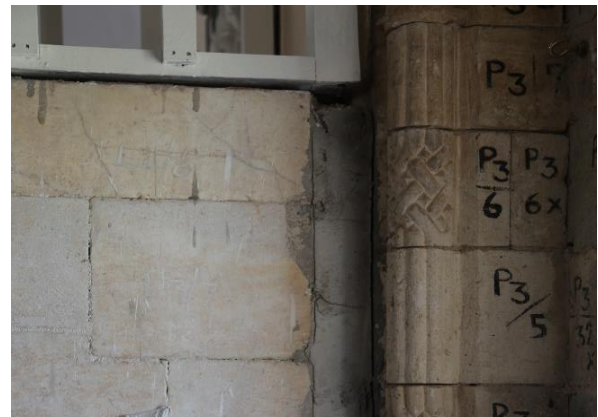
Figure 4. Stone wall joints problem in the interior.
