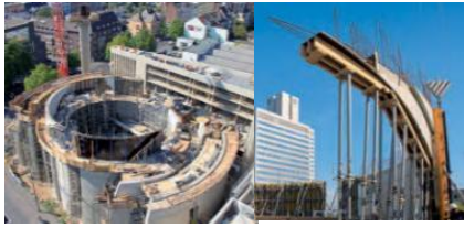
Figure 10. Several concrete shell segments gradually growing together and meet to form a cantilever [18]
