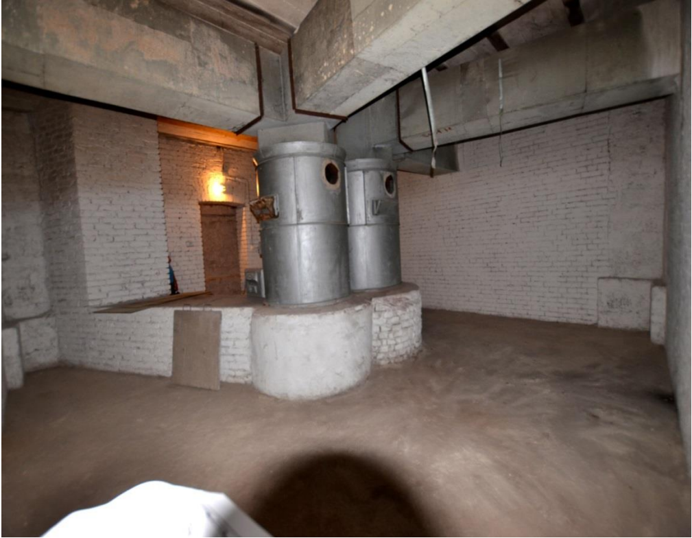
Photo 22: The Room of Heating Boilers Located in the Center of the Basement of Carol I (King) Mosque in Constanța
