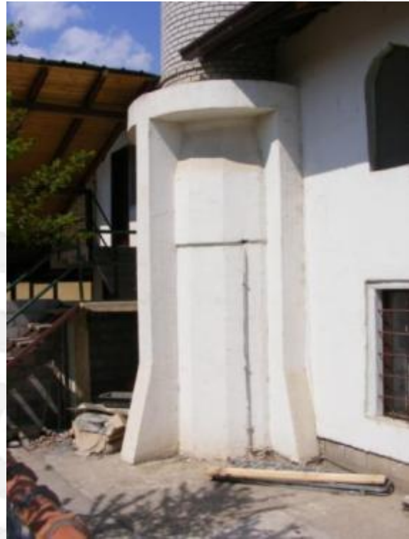
Fig. 1.9 Minaret view from south-west, the armored concrete part to the level of the mosque shed.
