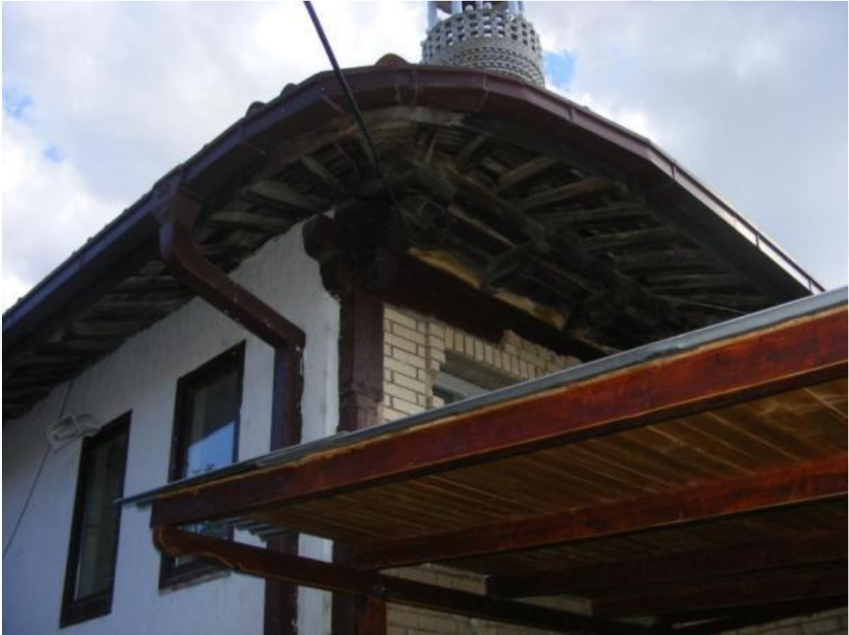
Fig. 1.27 Exterior view, the roof/shed of the new annex (down) and the sheds of the older annex (up).
