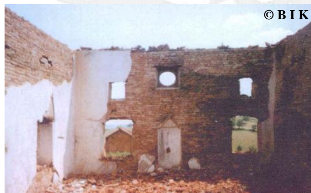
Fig. 4.5 Interior view of the after war (1999), the front or the kibla wall
