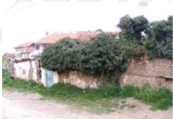
Fig. 1.5 Old wall parts from mud bricks on the street to the southwest of the KARAMANLI Mosque. Between the Mosque and the street there is the River TÈRRSTENA.
