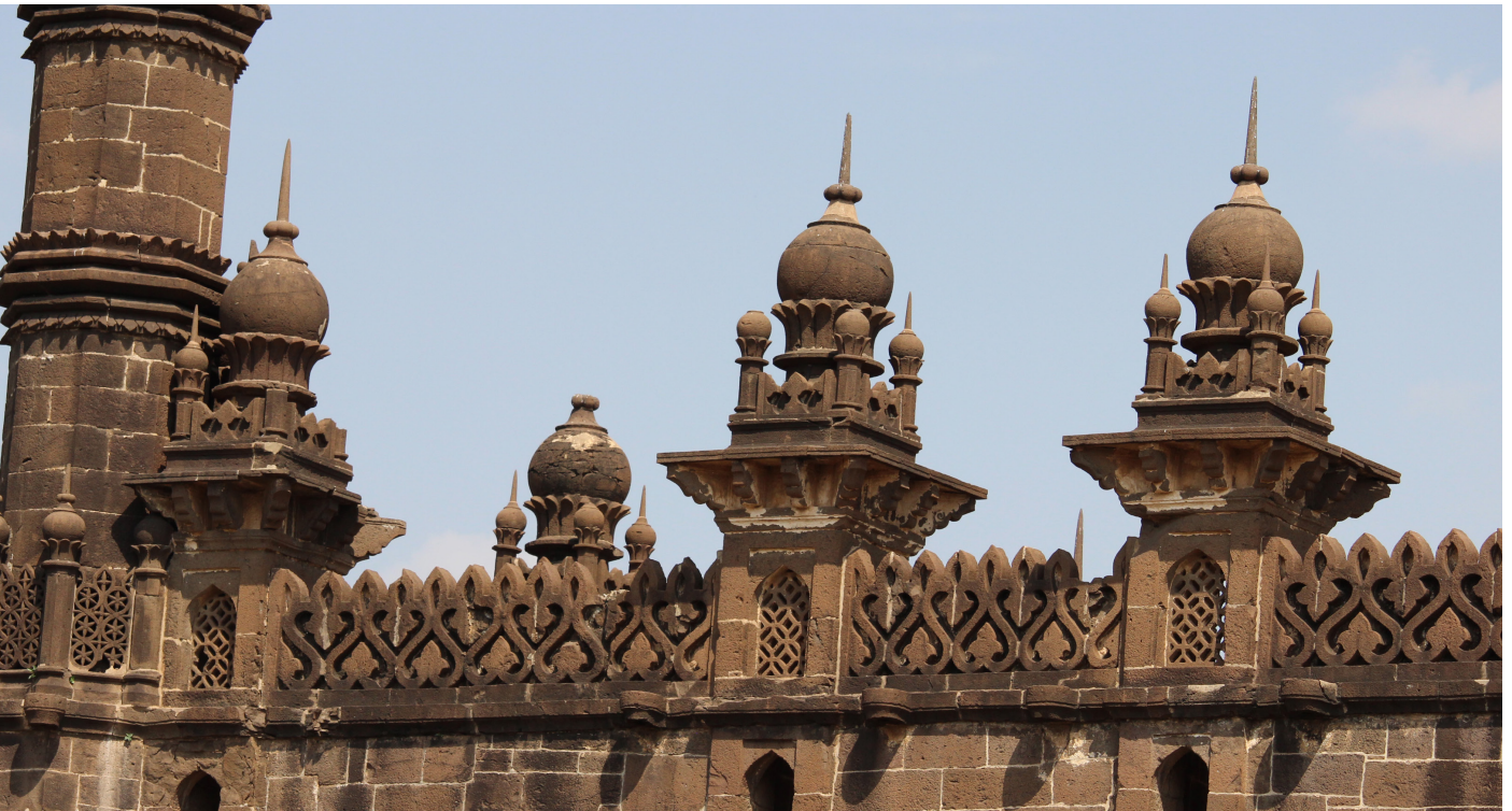
Parapet and finials in Ibrahim Rouza Complex, built in 1626 CE Location: Bijapur, India
