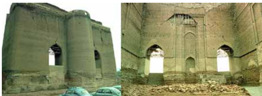
Fig. 19: Tabriz, Ali Shah Mosque, exterior from southwest and interior view from north of the qiblah wall showing the mihrab at the centre of the three relieving arches and the two openings at the sides.
