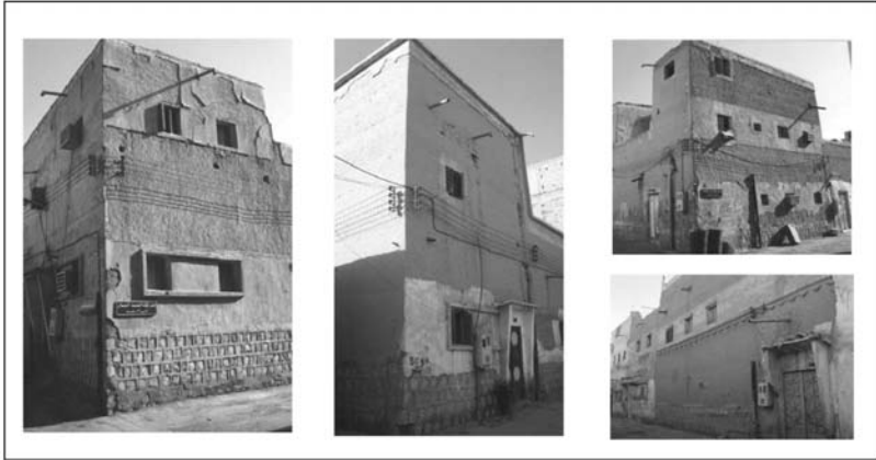
Fig. 2.6. The mud surfaces in the traditional houses in Riyadh plastered by cement and the traditional house gate was replaced by a concrete one because it reflects modernity. Source: Visual survey 1995.
