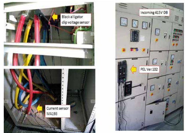
Figure 2: PEL instrument, sensors and electrical panel
