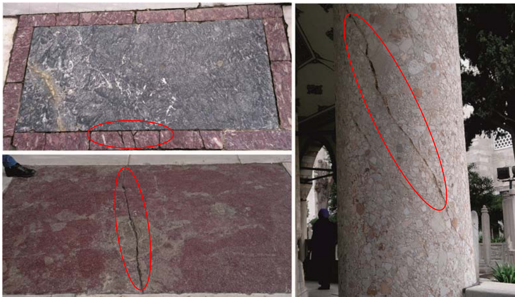
Figure 2. Crack deformations in different natural stones used in Suleymaniye Mosque
