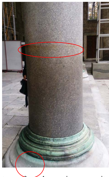
Figure 11. Remaining trace of metal corrosion on granite and marble surfaces
