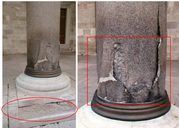
Figure 4. Alveolization (ellipse) and fragmentation (square) the view of granite column located in mosque courtyard
