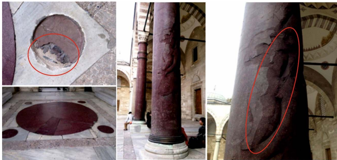
Figure 7. Cracking and loss occur with freeze-thaw effect on the porphyry column and floor
