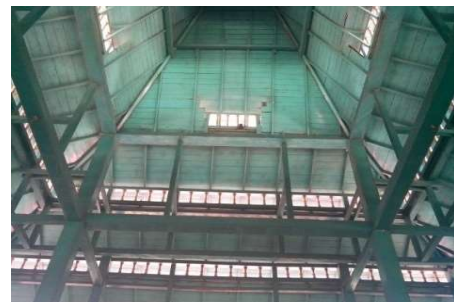
c. Roof ventilation (V1).
