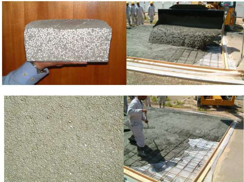
Figure 18. cross-section view of the final concrete/foam bubbles surface and the light-weight structure during production
