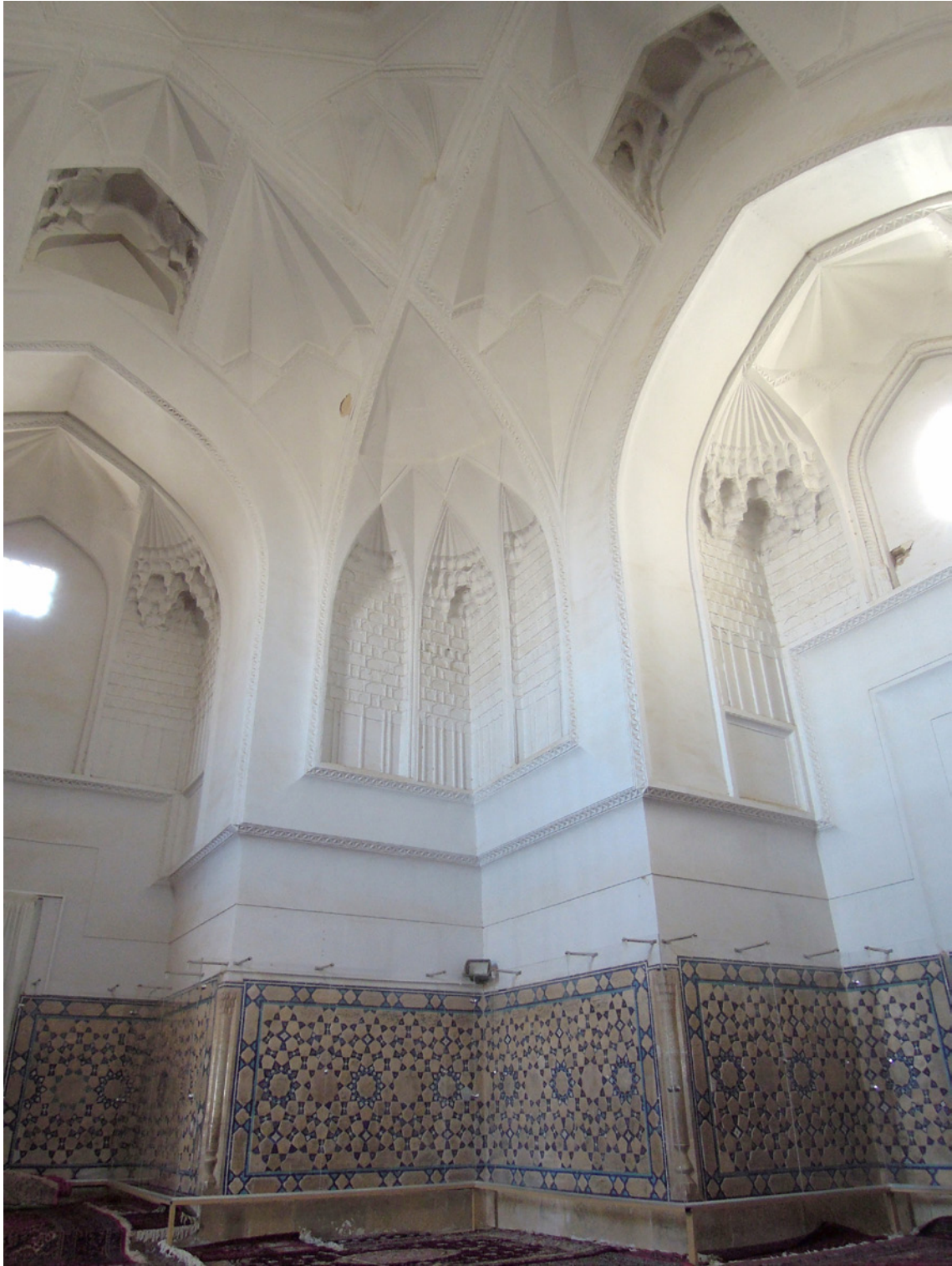
Fig. 35. Taybad, Zayn al-Din Mausoleum, dadoes in the main domed chamber. (Photo: Sandra Aube, 2015)
