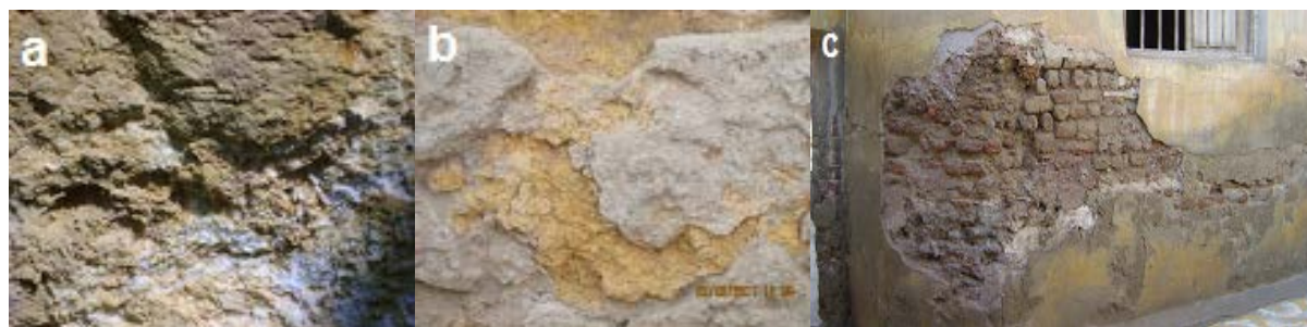
Figure 6. Photograph of decay features common at the Helal mosque. a—Efflorescence's to light-colored crust tracing the surface; b—Scars of flaking, c—Lost in brick, detachment of plaster and soiling by groundwater at the lower part of the mosque.
