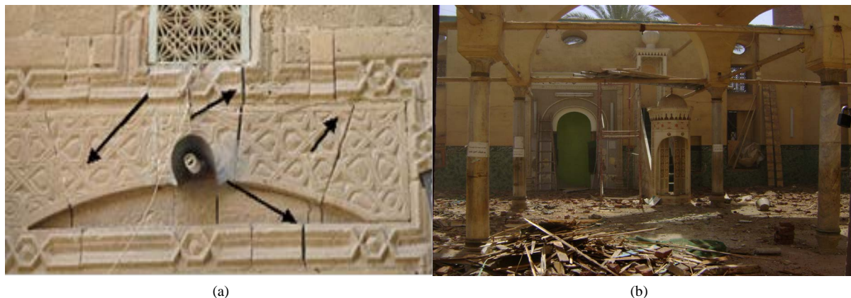
Figure 5. a—Cracks and macro cracks at the entrance of Helal mosque; b—Collapse of large parts of the ceiling of the mosque, especially north arcade.
