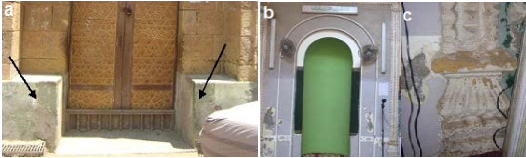
Figure 7. Old faulty restorations by Portland cement. a—Disappeared of Islamic decorations in the mosque façade by cement; b—Old restoration around mihrab which covered the decoration with Portland cement, industrial lacquers and carpet; c—The decoration was covered with lime and gypsum. Collapse of large parts of the ceiling of the mosque, especially north arcade.
