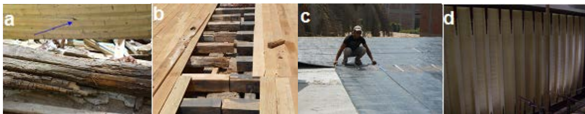
Figure 18. Restoration steps of the ceiling of Helal mosque. a—Deteriorated ceiling wood; b—New wooden panels during restoration process; c—Certekt layer; d—The ceiling after repaired.
