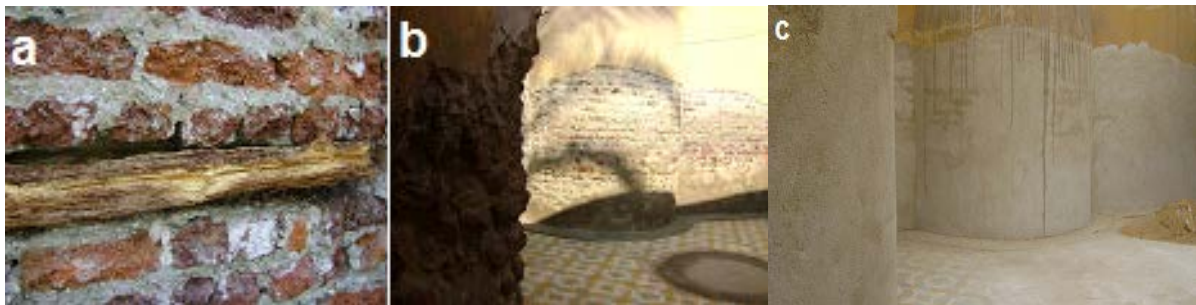
Figure 23. The restoration intervention at the brick walls. a, b—The brick wall after removing the deteriorated old mortar with salts; c—After restoration.
