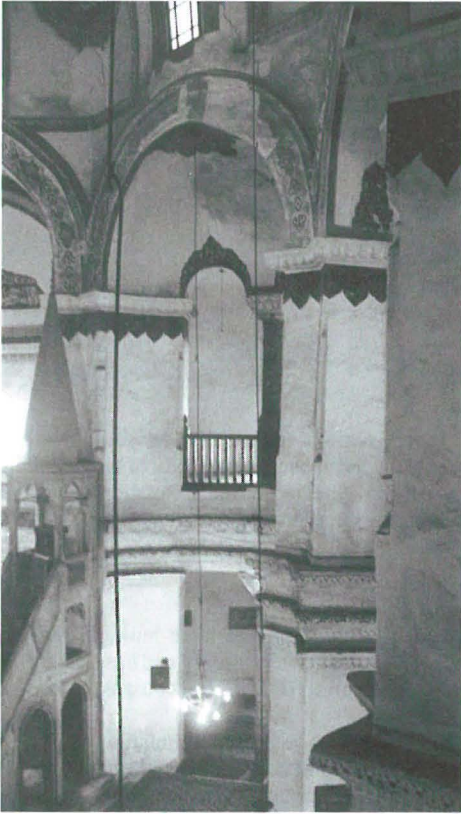
Figure 1. Deformation of piers.
