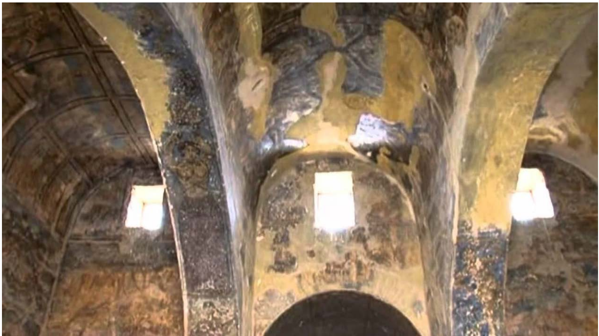
Figure 71: Qusayr Amra hall roof with three parallel barrel vaults Source: Mohammad Abu Omar
